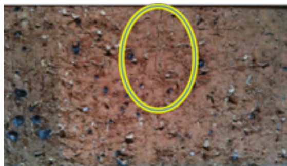
Superficial face crack that does not penetrate to the core (above right)
