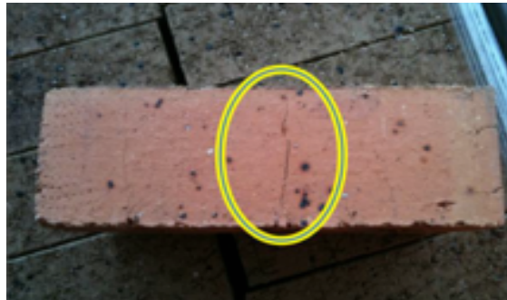
Cracks in the back of the brick
